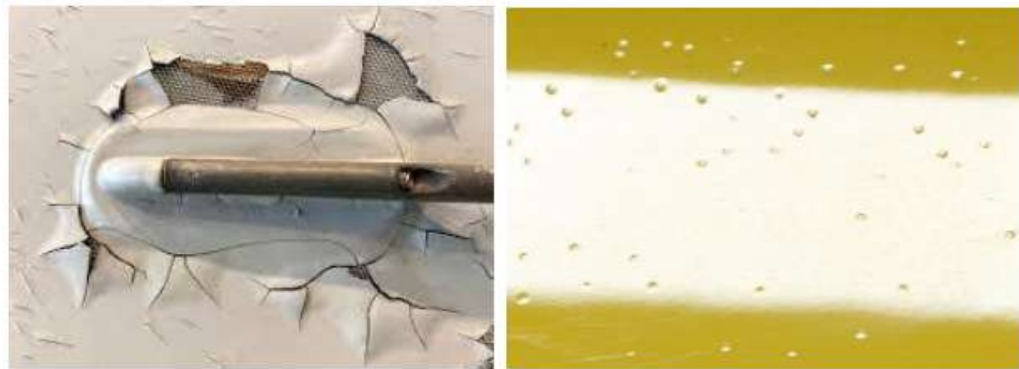
Gambar 3. Peeling Paint Defect & Solvent Pop Paint Defect
