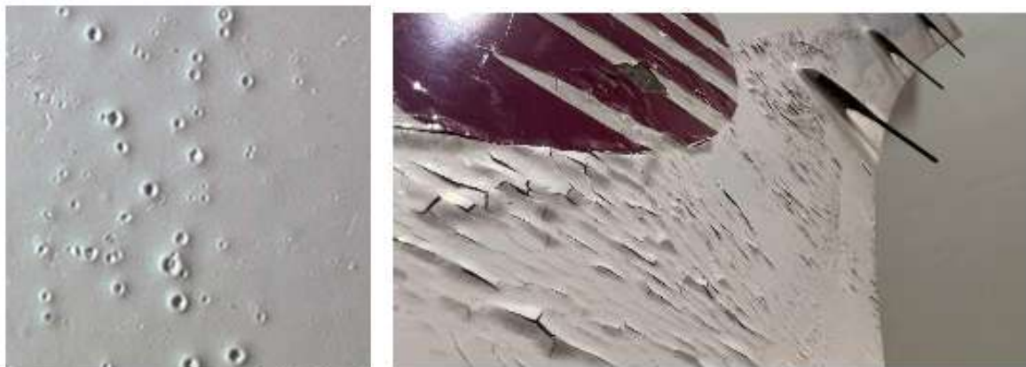
Gambar 4. Fish Eye Paint & Cracking Paint Defect
